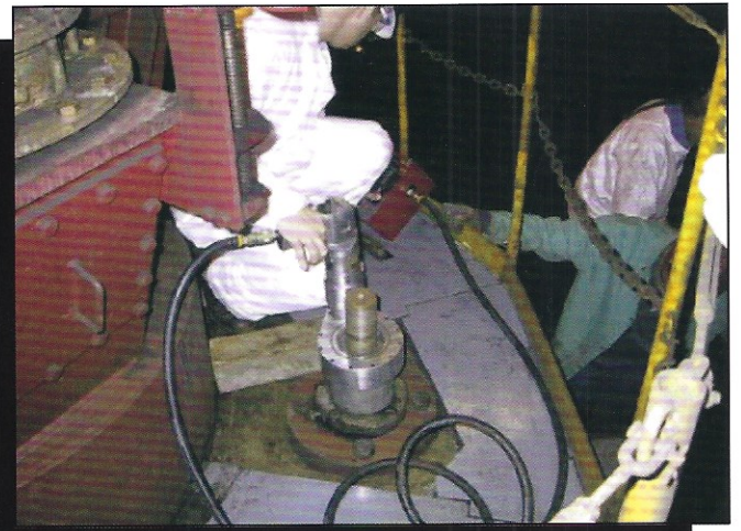
Tension Adjustment Bolts on Ball Mills
